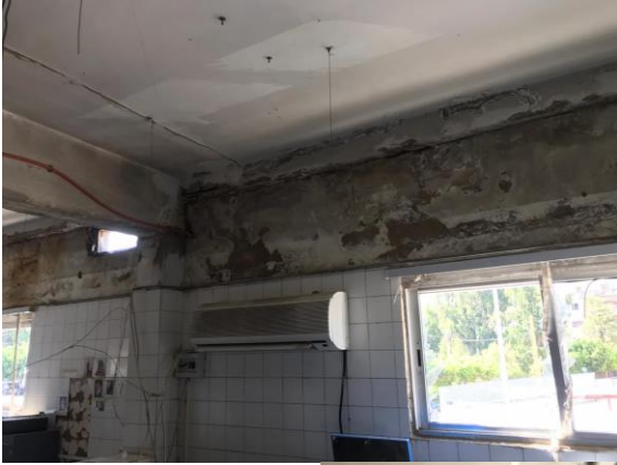
2-A : Old building ceilings don't exist
