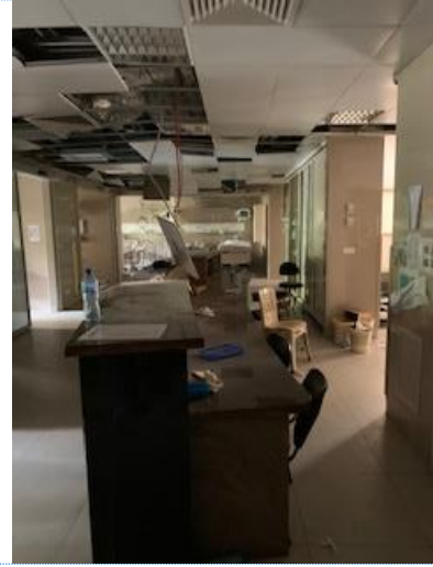
Complete damage of the unit ICU
